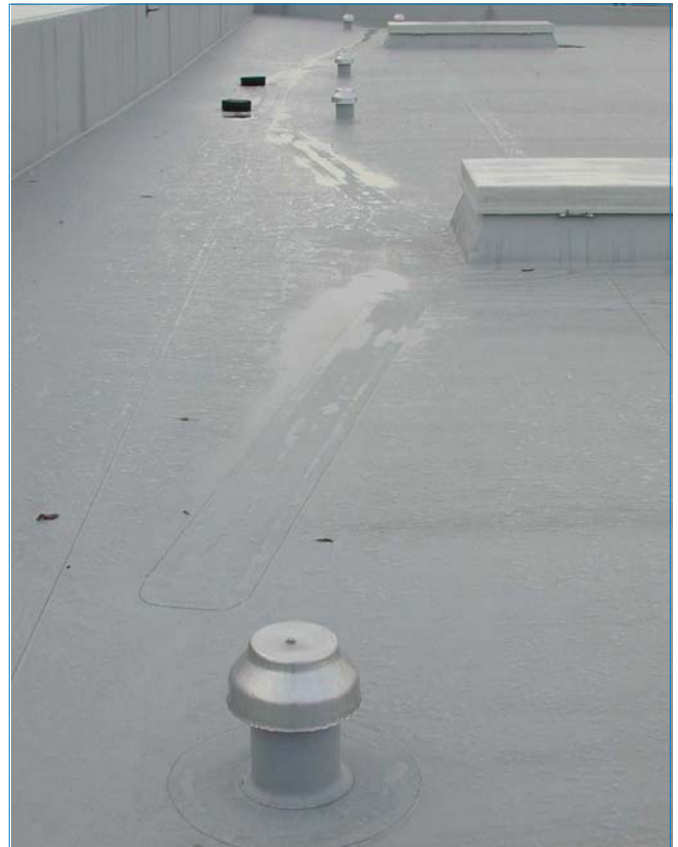
Vacuum vents in perimeter zone
